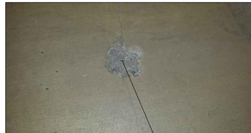
TYPE 2: EXPOSED CONCRETE NO REBAR EXPOSED (at second floor of parking deck) Not to scale Concrete spalled (Refer to spall repair details on sheet S-3)
