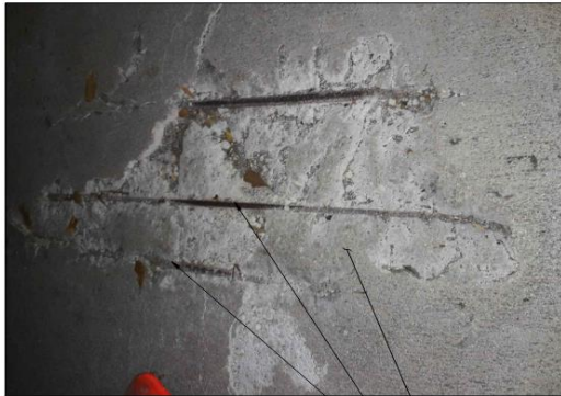
TYPE 1: CONCRETE SPALLED WITH REBAR EXPOSED (at second floor parking deck) Not to scale Concrete spalled (Refer to Type 1 Repair Detail on sheet S-3) Exposed rebar
