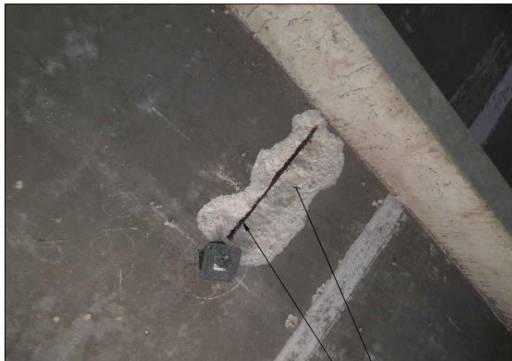
TYPE 1: CONCRETE SPALLED WITH REBAR EXPOSED (at bottom of parking deck) Not to scale Concrete spalled (Refer to Type 1 Repair Detail on sheet S-3) Exposed rebar
